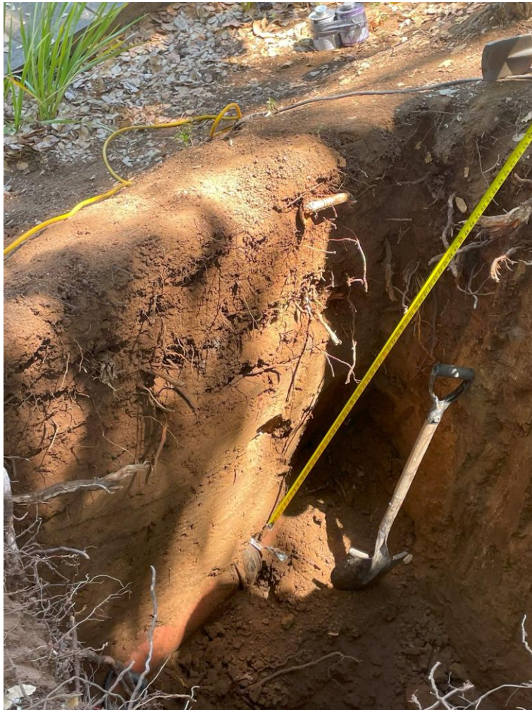
Exhibit 1: Point Repair at La Loma Dr
